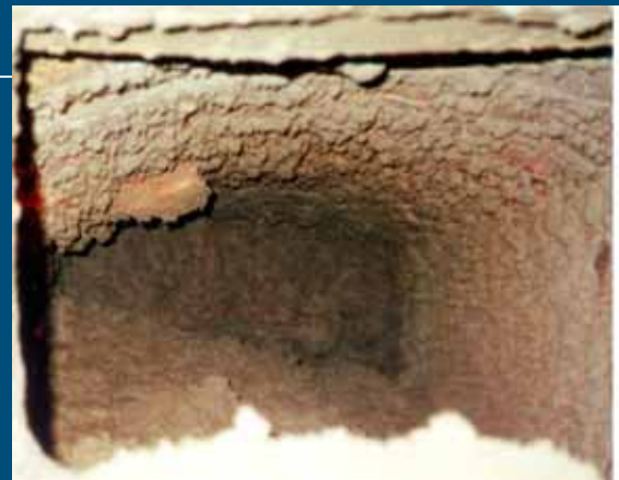
Fouling on the furnace walls
